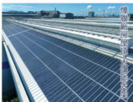
Solar energy stand-building of YIEH UNITED STEEL CORP.
